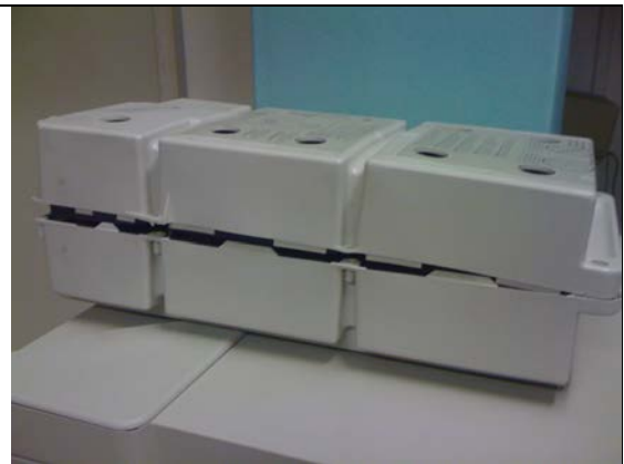
One of the broken batteries modules.
