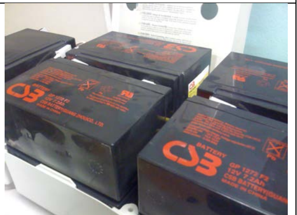
Deformed batteries inside a batteries module.
