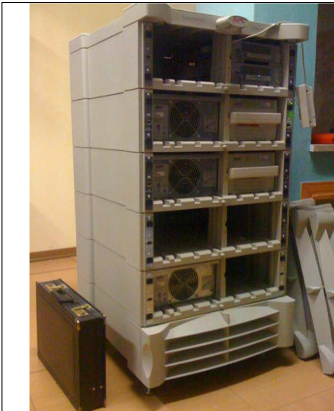
Big UPS, modular, in the left column the power modules and electronics, in the right column the batteries modules.
